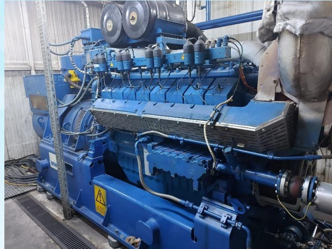
Figure 1. Natural gas-powered generator
