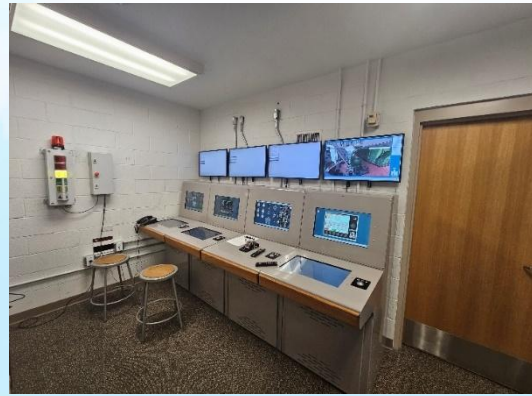
Figure 4 ERS 2 FMS Engine Control Room
