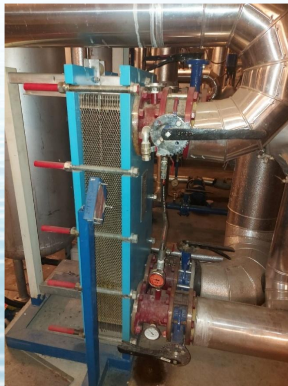
Figure 2. Jacket water-hot water heat exchanger
